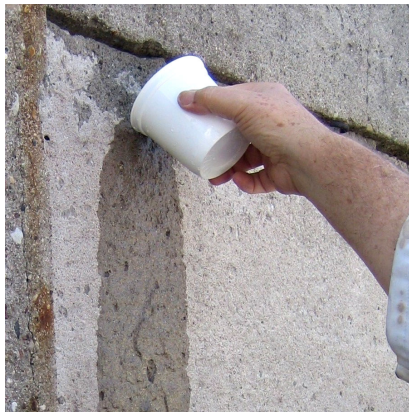
Water on UNPRIMED wall is adsorbed
